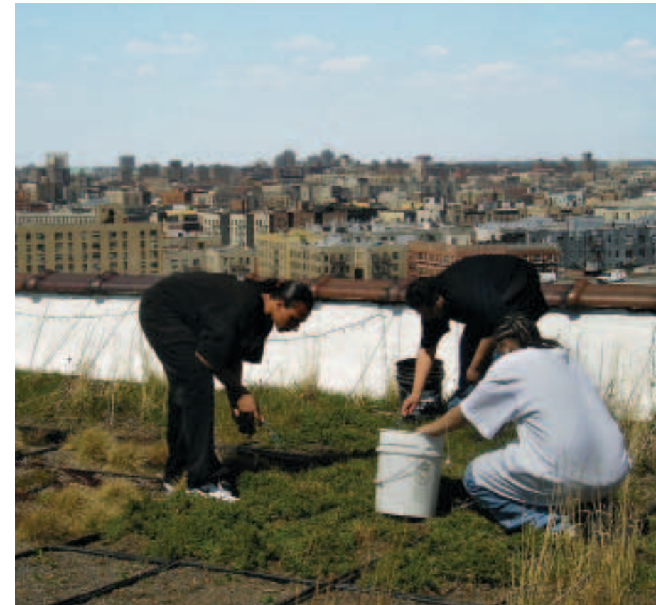
Green collar workers from Sustainable South Bronx turn a rooftop into a green roof.
